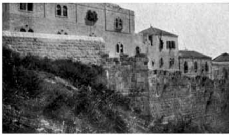
No. 35. The Rampart Walk covered with 12 ft. of "tip," and showing a new wall built on top of the "tip."
