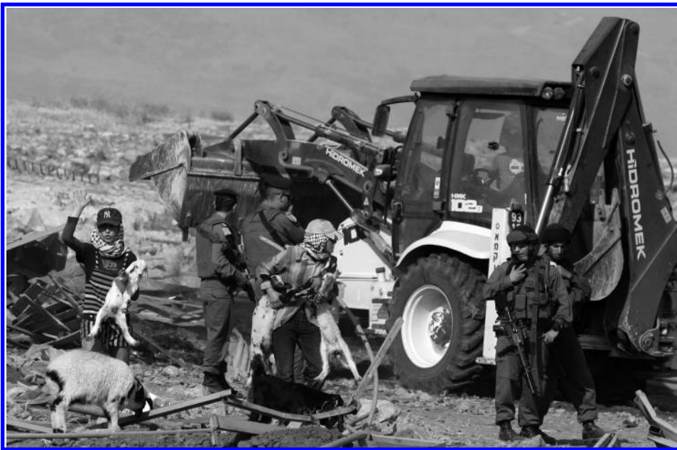
Bedouin evacuate livestock as the Israeli military demolish their homes and structures in the village of Hadidiyya, located in area C of the West Bank on 21 June 2011. (Saif Dalah/AFP/Getty Images)
